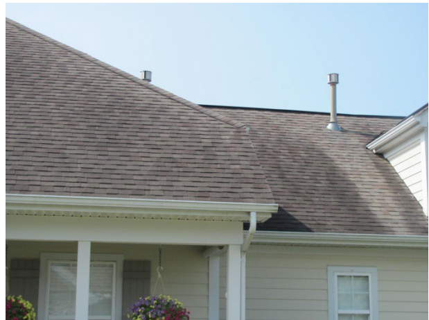
Weathered shingles at Unit 400
