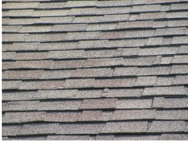
Granular loss evident at shingles at Unit 600
