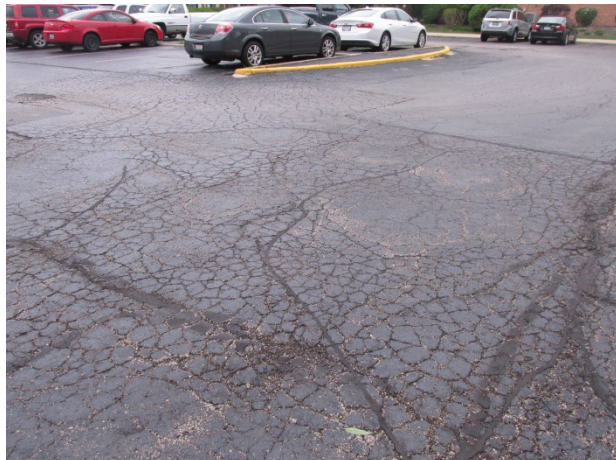
Alligator cracks adjacent to recent patch repair
