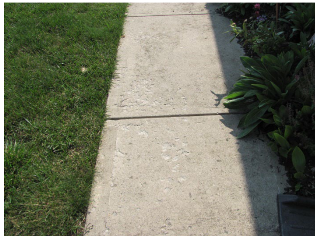
Spalled concrete sidewalk at Unit 200
