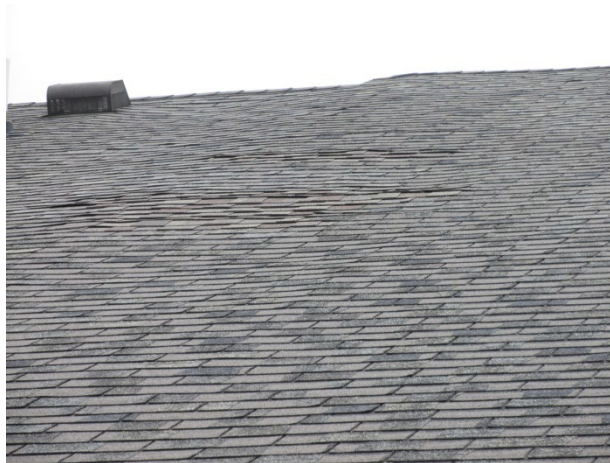
Sheathing deflection evident at Unit 700
