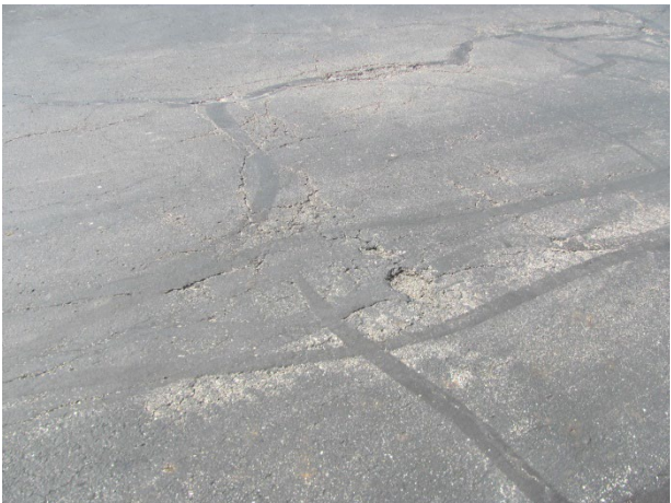
Pavement raveling and onset of potholes
