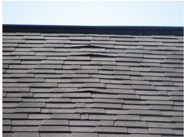
Lifted shingles at Units 200 and 201
