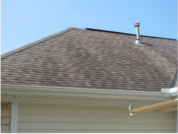
Weathered shingles at Unit 500
